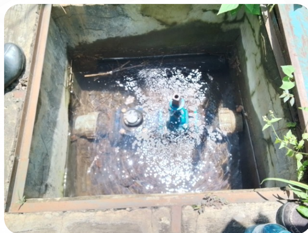
Figure 1: Leaking valve contributing to NRW
