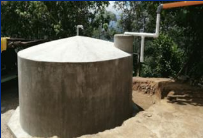
Figure 6. Ferrocement cistern for rainwater harvesting
