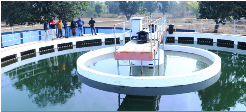
Filtration Plant of GMVRWSS at Sontola village, Harrhatola Gram Panchayat, Gohparu Panchayat Samiti, dated 10 th February 2024
