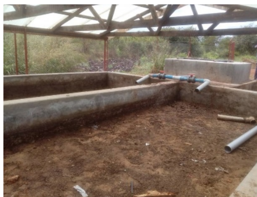
Photo 1: Faecal sludge treatment plant
